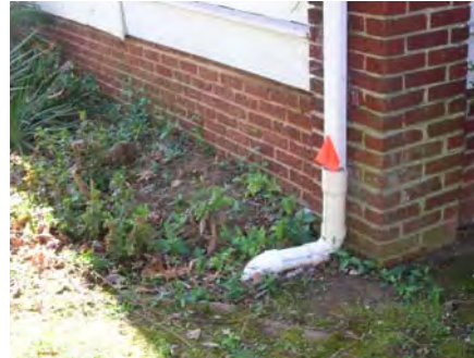
Prohibited downspout connections can overload sanitary sewers with stormwater and contribute to overflows.
