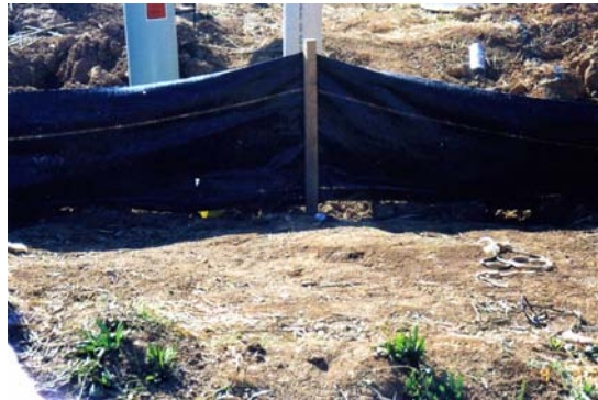
Silt fencing should be buried to stop water, mud or dirt from leaving a construction site. This fence is not buried. You can see underneath it!
