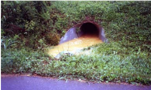
Brown water should NEVER leave a pipe. This is illegal.
