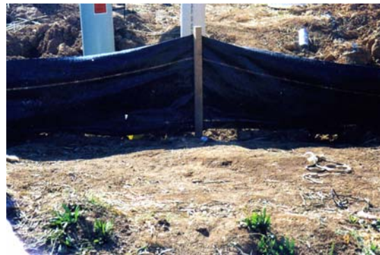
Silt fencing should be buried to stop water, mud or dirt from leaving a construction site. This fence is not buried. You can see underneath it!
